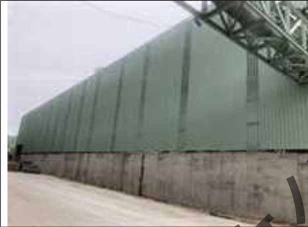
封闭式炉料棚
